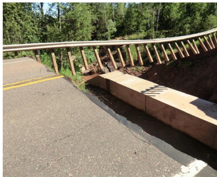
More and more rainfall in Northern Wisconsin is being delivered in heavy events as the climate changes. U.S. Highway 63 northbound, east of Grand View at the Twentymile Creek stream crossing on July 11, 2016. Photo credit: Andrew Teal
